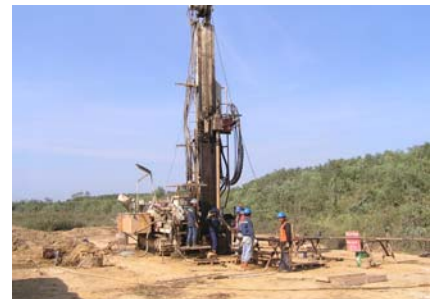
Deep hole drilling program continues to delineate reserves at the Tutupan mine
