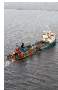
Dredging of the Barito River sea channel in November 2008 by the trailer dredge Ham 312
